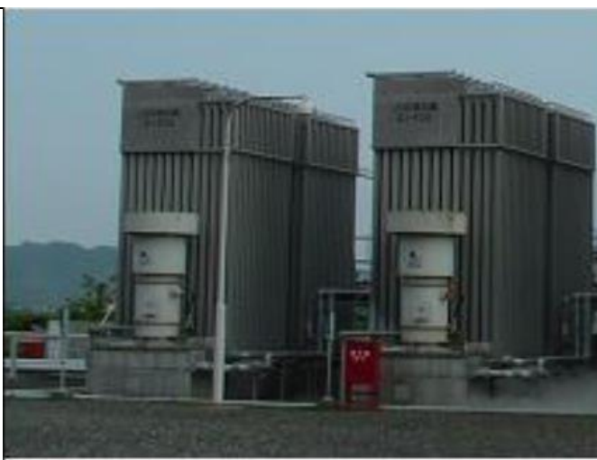
Figure 6: Ambient Air Vaporizer (Source: BV 2009)
